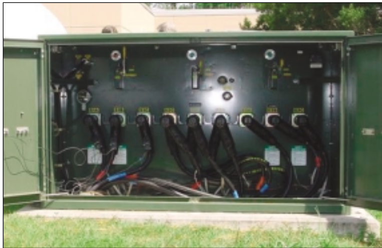
VFI pad-mounted switchgear greatly improves reliability
