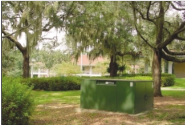
The low profile equipment is aesthetically pleasing in this campus setting
